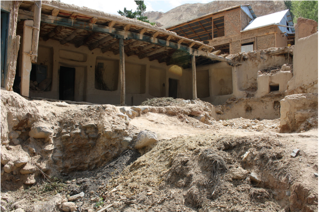
Damage from mudslides in Ayni District, 2010
