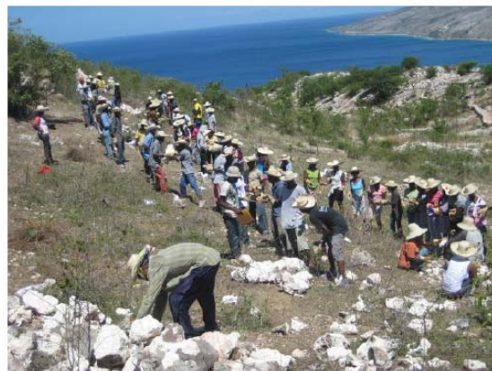
A line of workers gather piles of rocks to build retaining walls on a hillside above Blockhaus, Saint Marc.
