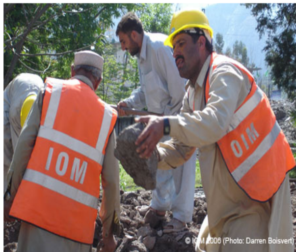
© IOM 2006 (Photo: Darren Boisvert) A mountain to move, one rock at a time. Locals in Muzaffarabad begin to clear the rubble so public buildings can be rebuilt.
