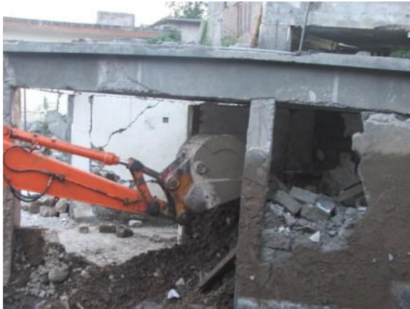
Fig 1.2 Clearing the slide damage from inside the house
