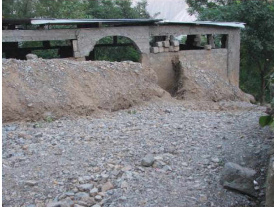
Fig 1.3 Chela Bandi Mosque before clearing
