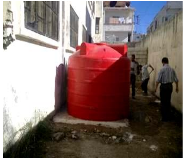
IOM installed water and sanitation facilities in a public shelter where 30 IDP families are living in Lattakia. © IOM 2013 (Photo: IOM Syria).
