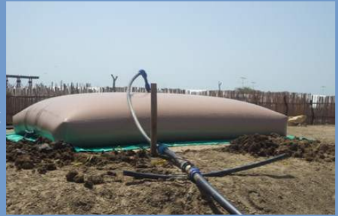
IOM-installed water bladders provide access to clean water in the new extension site
