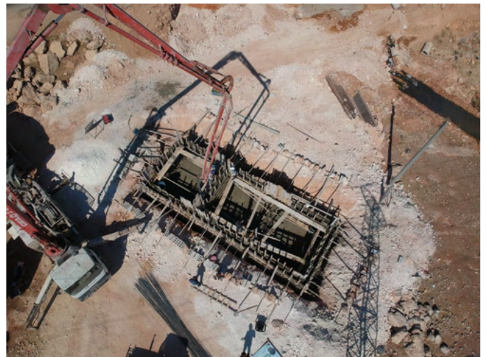
Construction works of multi-chamber septic tank in an IDP site in Idleb – Northwest Syria © IOM 2020, through WATAN Foundation.
