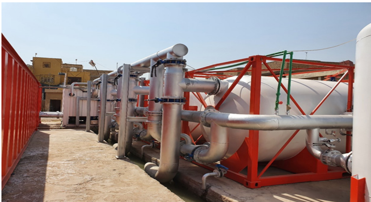
Al Ghadeer water complex providing long-term safe access water for 24,000 beneficiaries © IOM Iraq, 2021
