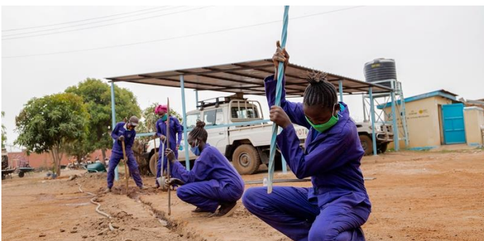
Youth in South Sudan working on solar panel installation supported by IOM © IOM/Muse Mohammed
