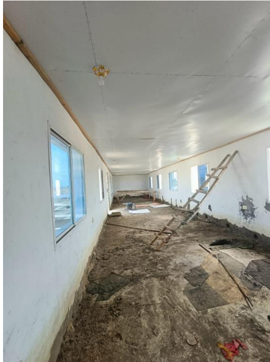
Photo 1: Interior of the Filter Gallery Control Room
