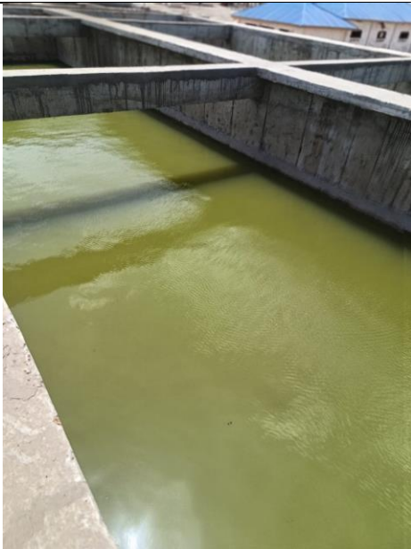
Photo 5: Flooded sedimentation tank
