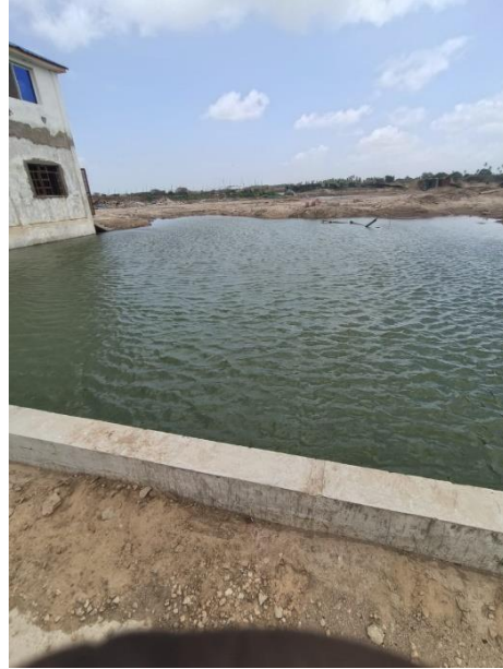
Photo 4: Flooded area at the excavated area around the pump house and clear water tank
