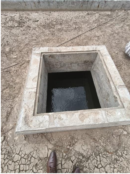
Photo 3: Water filled 1000m 3 Clear Water Tank
