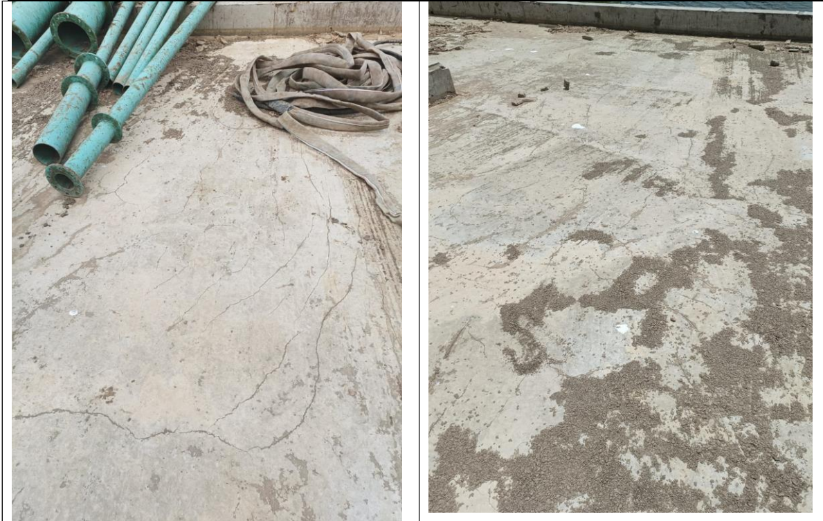
Photo 2: Cracks at top of Roof Slab on 1000m 3 Clear Water Tank
