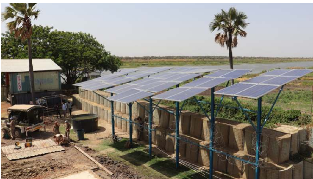
IOM monitors the environmental performance of its offices worldwide through environmental inventories. Shown here: a solar energy system is used to pump half a million litres of water from the Nile River daily to supply water to the Protection of Civilians site and the Humanitarian Hub in Malaka, South Sudan (this solar system was not funded with unearmarked funding). © IOM 2020/Angela WELLS
