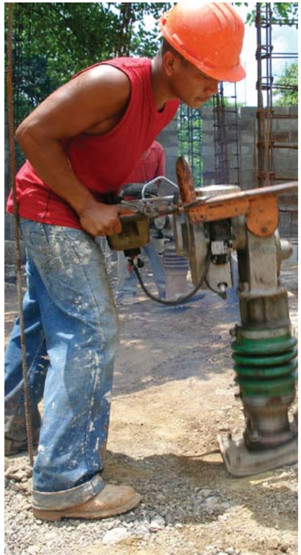
Nicaraguan migrants in Costa Rica working in the construction industry. (Photo: © Jéssica Saavedra/IOM 2007/MCR0003)
